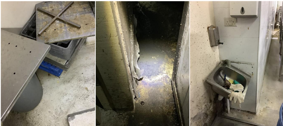
The premises was found to be poorly maintained with pest infestations. (Photos: SFA)
