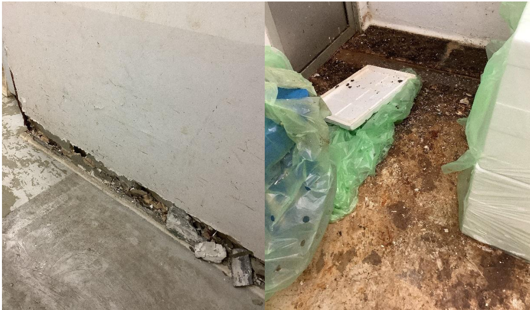
Badly damaged wall in processing area (left) and poor cleanliness condition of floor and wall in processing area (Photo: SFA)
