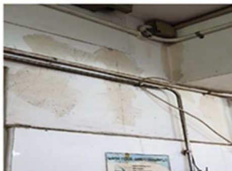
The premises had dusty walls as a result of poor housekeeping (Photo: SFA)
