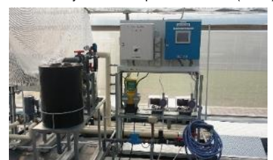
Smart fertiliser dispensing and self-filling water top up system
